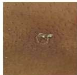
f) partially removed scab
